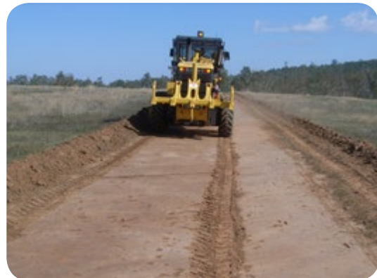
Scalping using a grader removes approximately 75mm of soil including much of the soil seed bank, which is windrowed to the side. In this example, a gentle spoon drain or furrow is created that harvests rainfall from the surrounding area to the centre providing long lasting weed control and water harvesting in one action. This high disturbance preparation method should be used very cautiously. Avoid sites prone to soil erosion such as duplex soils with a shallow sub-soil (B horizon) or sites with good native plant cover. It is best used in flat to gently sloping weedy sites with limited native groundcover.
